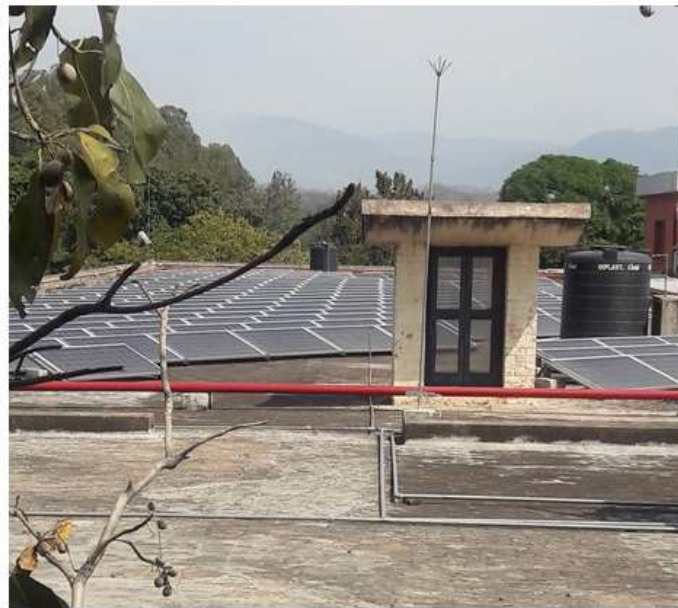
Solar Water Heater on roof of Boys' Hostel
